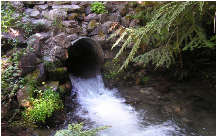
Example of a culvert that blocks fish passage and doesn't facilitate movement for terrestrial wildlife. Photo courtesy of Washington Department of Fish and Wildlife
